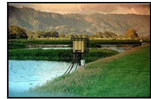
Biological Water Treatment Facility
